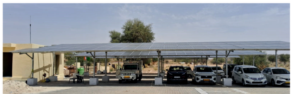
100 KW off grid SPV Power Plant (Car parking type) installed at Laungewala Yudh Sthal, Jaisalmer
