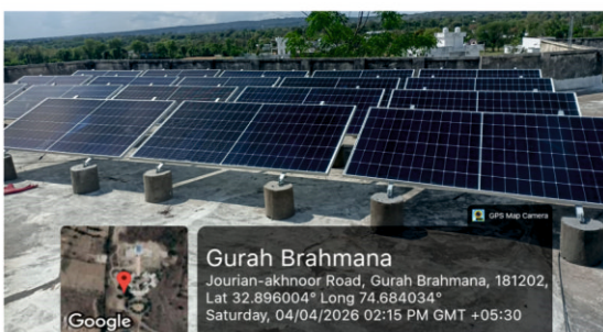
SPV Power Plant(s) installed at Govt. Buildings, J&K
